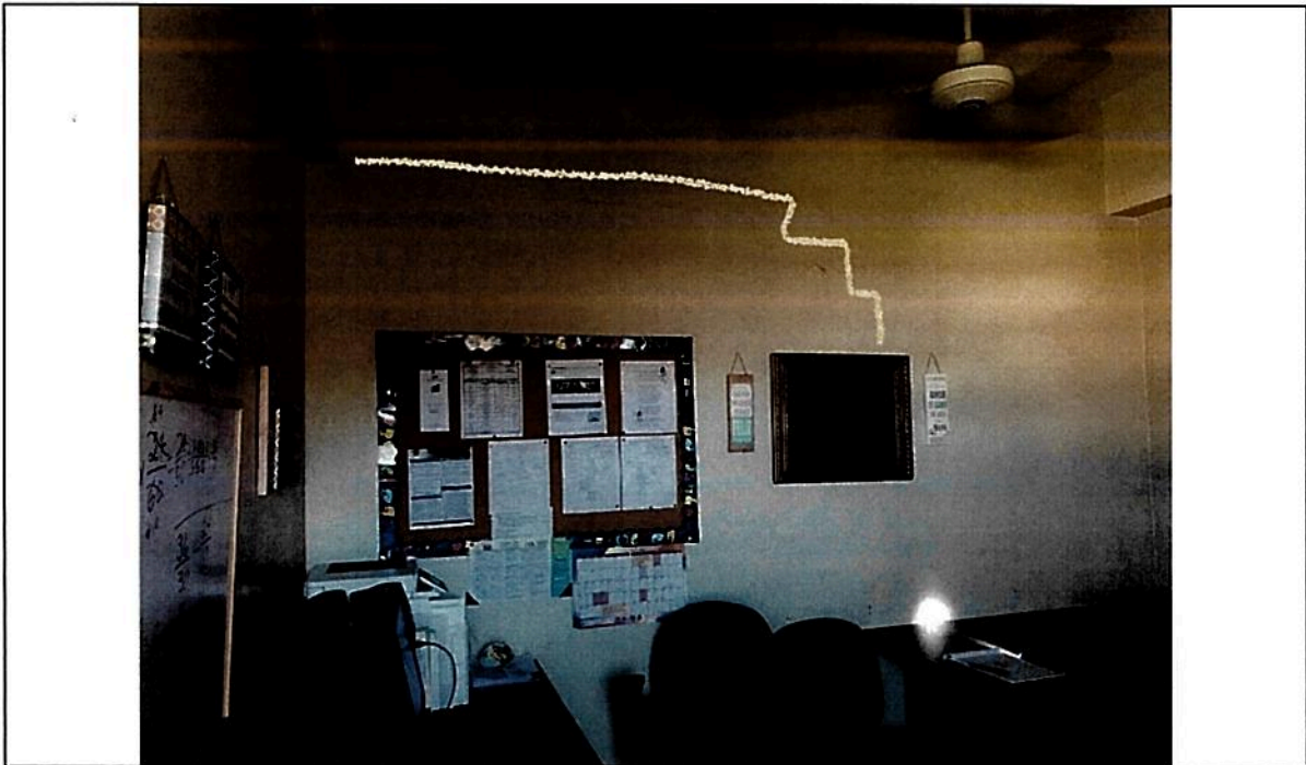
Picture 13 - Division wall stair step cracks at walls in classroom (ciencia ambiental) and small office (educacion especial) both on level 3
