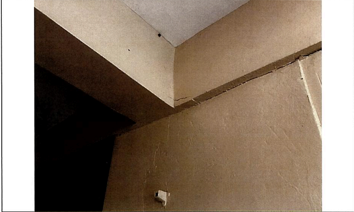
Picture 18 - Horizontal separations or cracks at division walls joints with ceiling slab, beams, or other horizontal component
