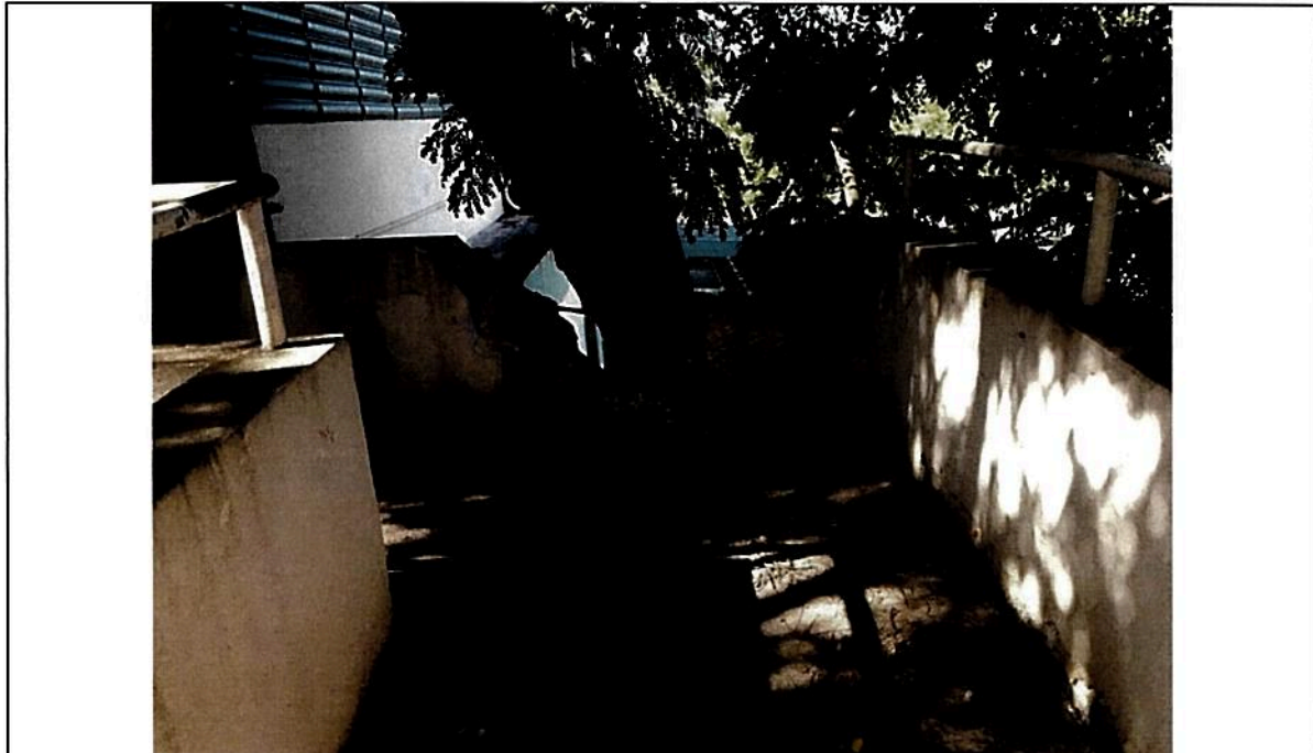
Picture 12 – Handicap Ramp reinforced concrete wall broken section by a falling tree during H. Maria. Strong impact along the long axis of the ramp by the tree.
