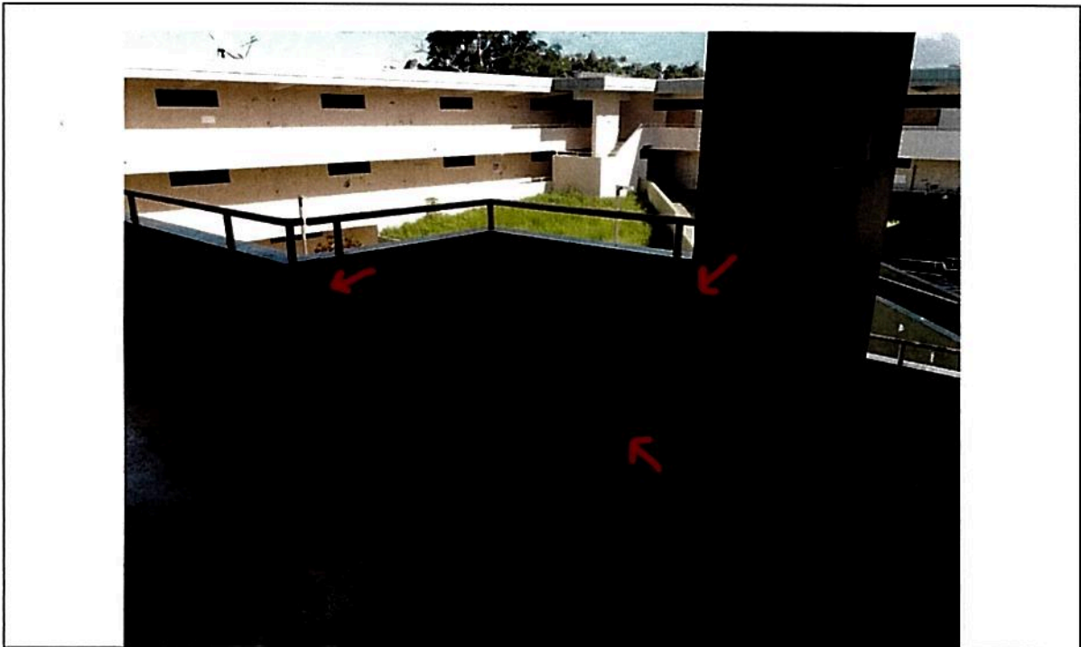
Picture 20 - Cantilever slab section on NW Stairs showing signs of separation and/or cracks related to the joint with the building and its' cantilever condition.
