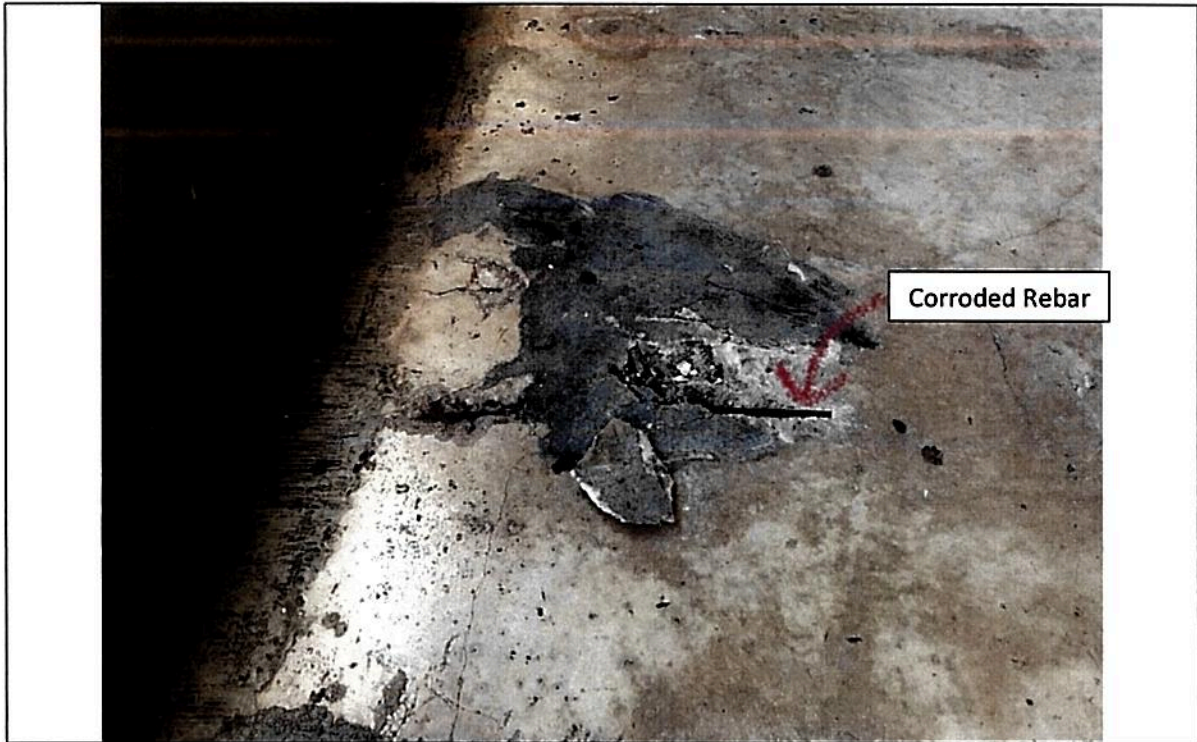
Picture #15 - Concrete Delamination or Spalling at borders of elements or local areas
