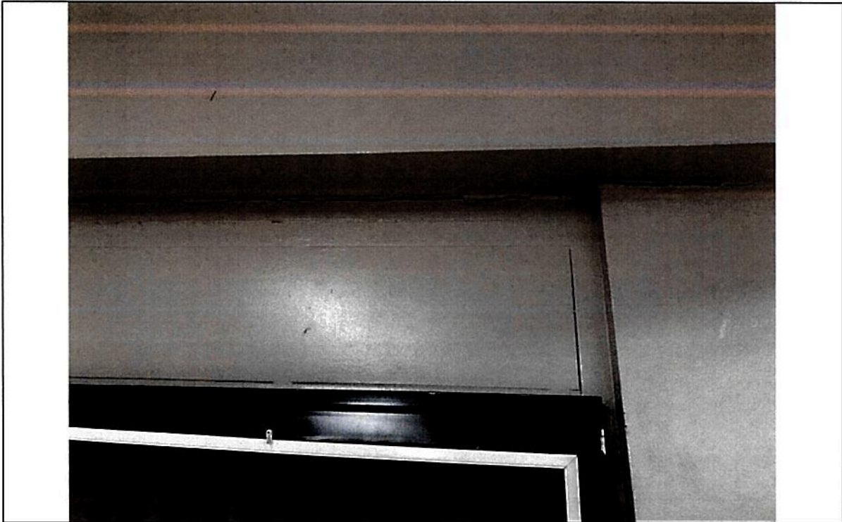
Picture 17 - Horizontal separations or cracks at division walls joints with ceiling slab, beams, or other horizontal component
