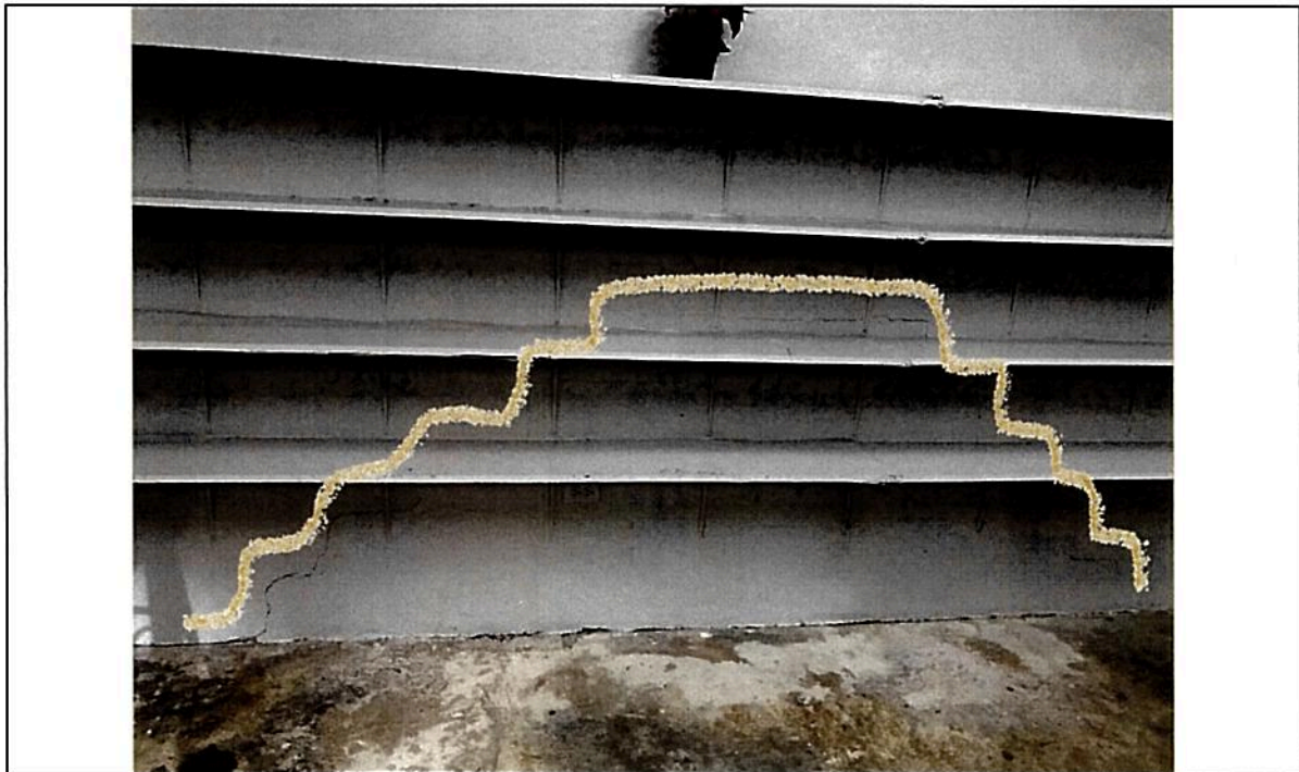
Picture 6 – Stair step cracks at least at two CMU walls segments in the vicinity of the SE building expansion joint (dining hall/corridor wall) – Image shows dining hall side
