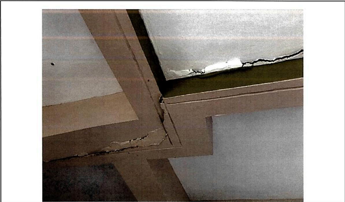
Picture 9 - Open construction joints between building modules (Cracked and loose plaster)
