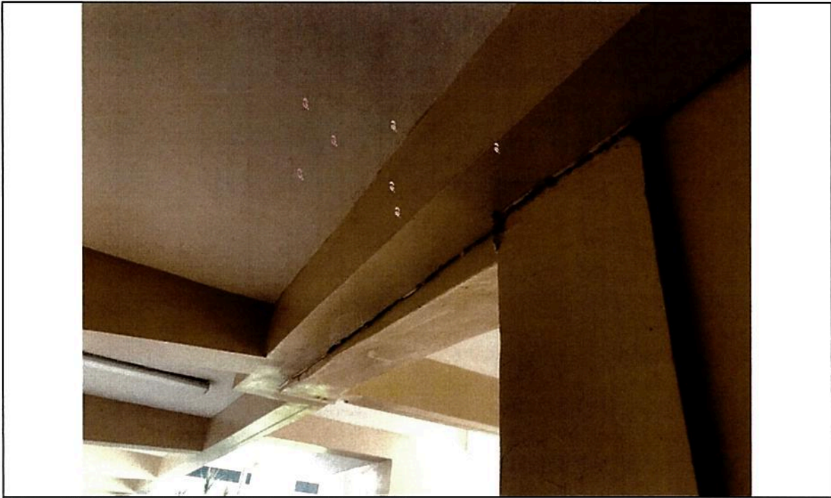
Picture 10 - Open construction joints between building modules
