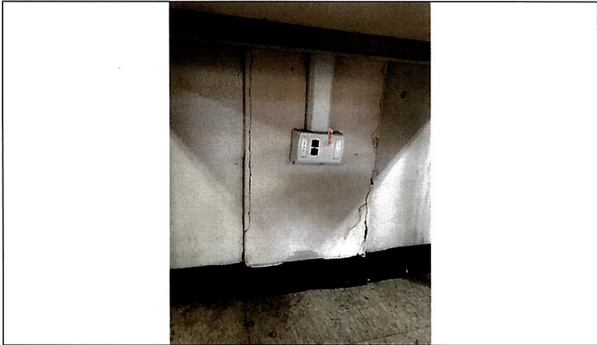
Picture #14 - Concrete Delamination or Spalling at borders of elements or local areas
