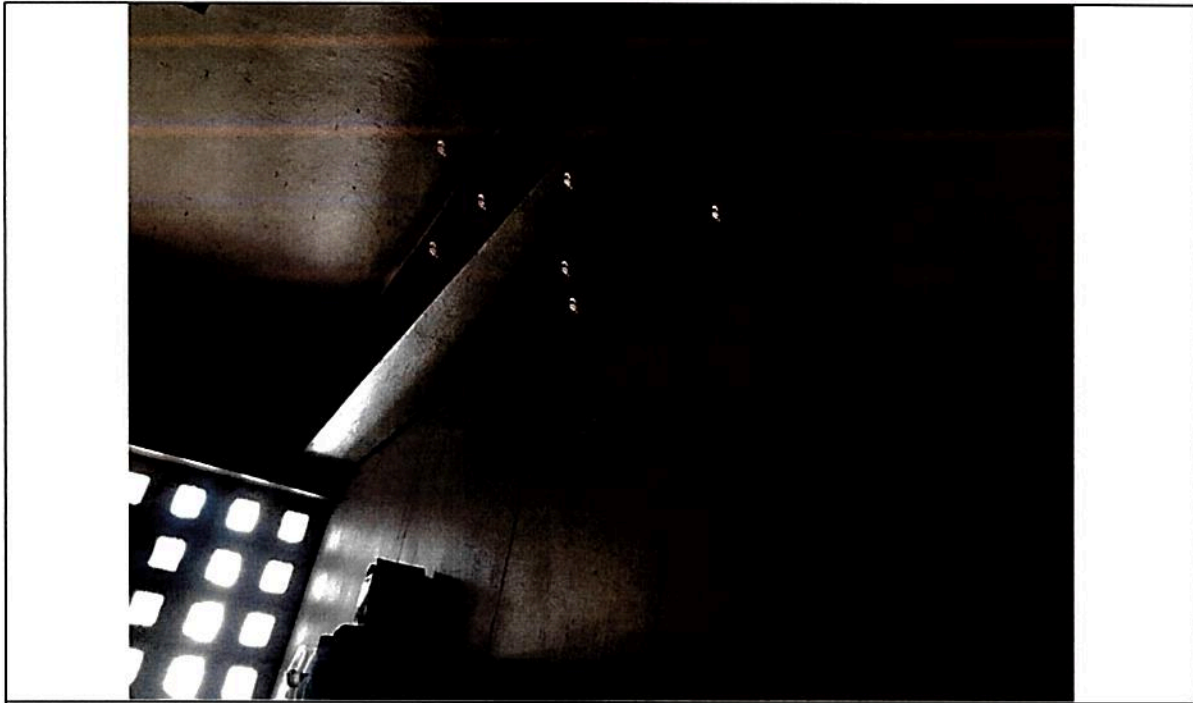
Picture 11 - Open construction joints between building modules
